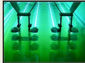
UV disinfection system
